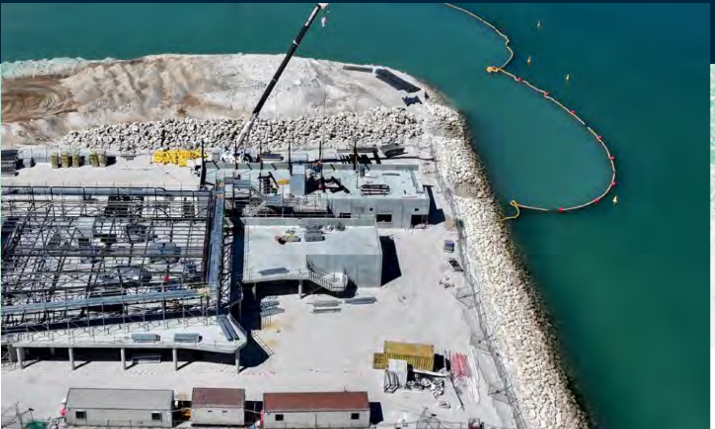
An aerial view of the new ORSSC building (front) and MRW (back).
